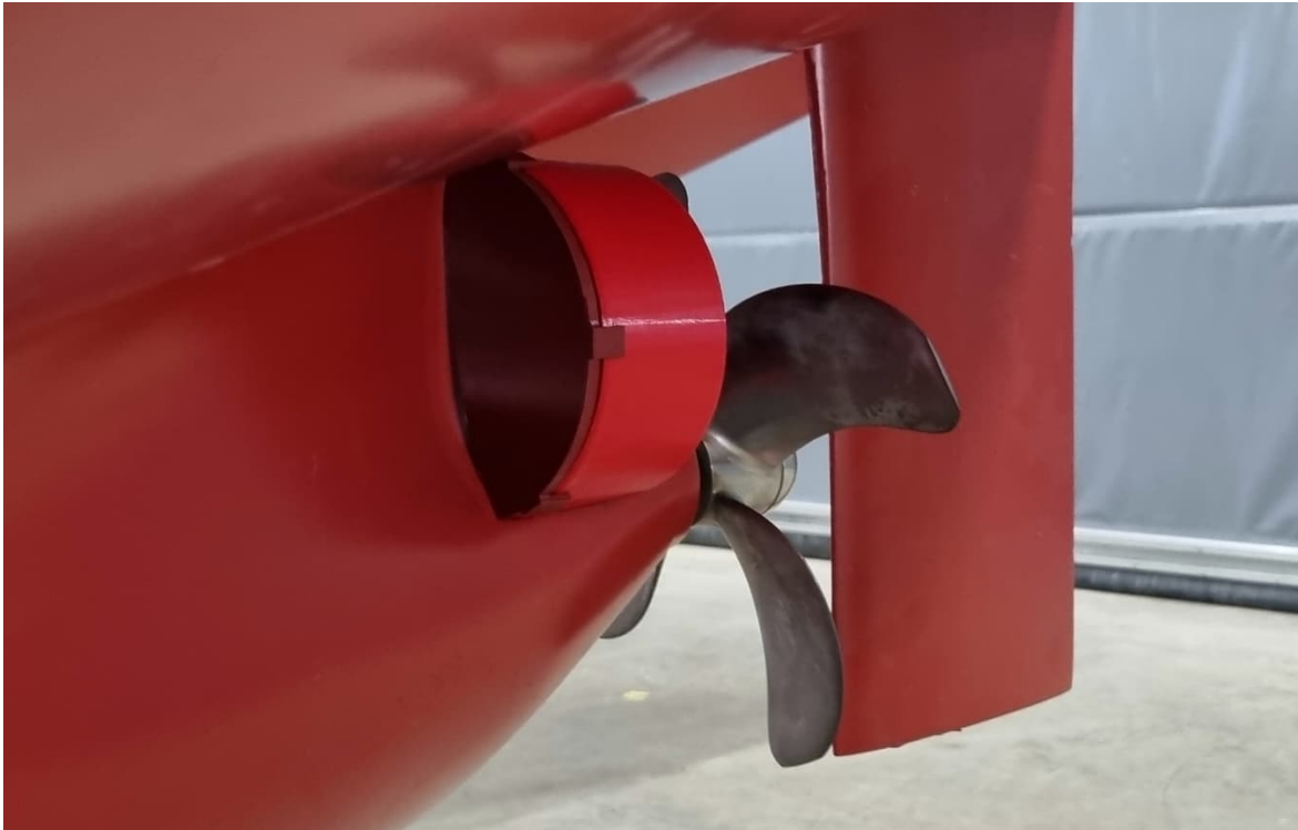
Figure 3-6: The Schneekluth -type duct 50% clogged. In 100% clogged situation the starboard side is also clogged.
